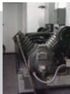
Air Compressor – Full Visible
